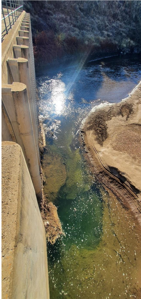
Figure 11. The intake as viewed from above. Sedimentation buildup can be seen at the intake
