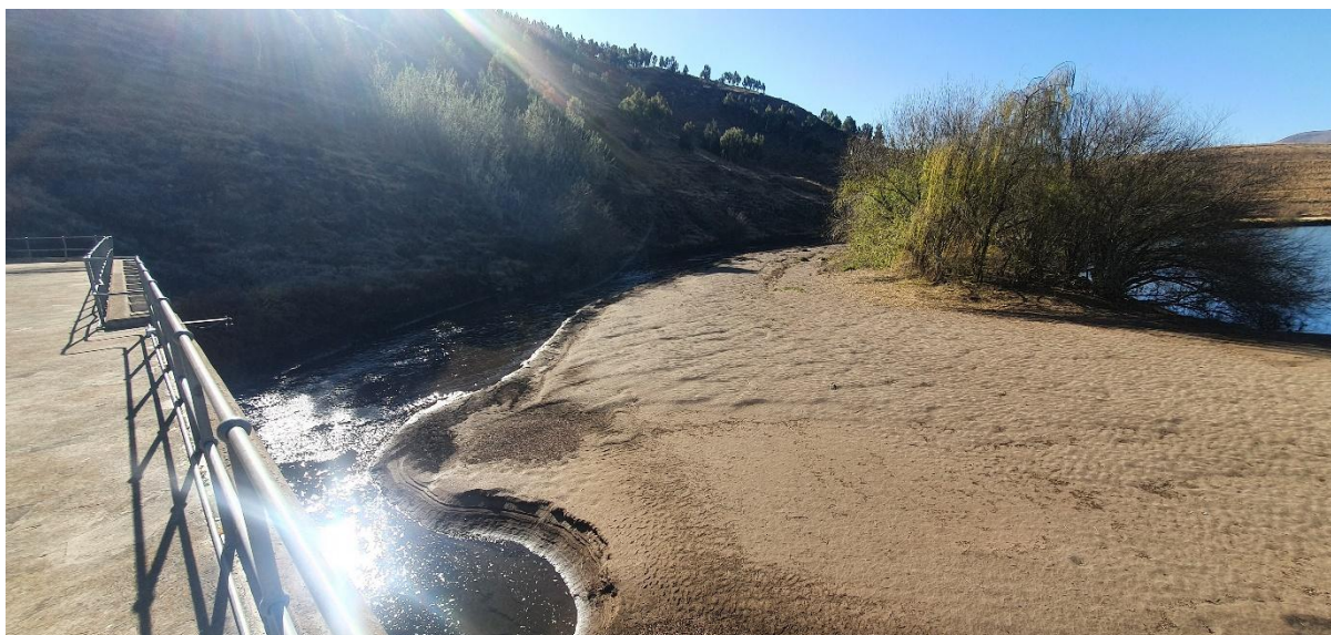
Figure 21. Sediment buildup in the river in front of the screens. The upstream end of the river can be seen towards the centre of the photo.
