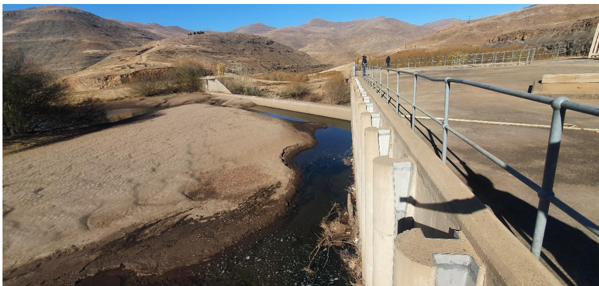
Figure 20. Sediment buildup in front of the inlet structure and weir. Handrails are installed around the platform for safety.
