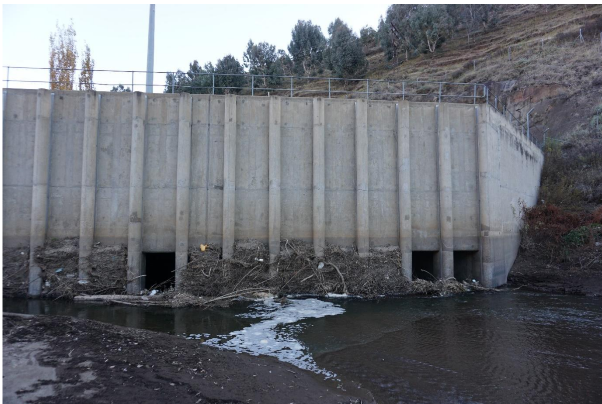
Figure 12. The intake structure as viewed from the river where sedimentation buildup has occurred. Flow through the screens is completely restricted by densely compacted debris with the screens of three screen bays removed to allow flow into the intake structure.
