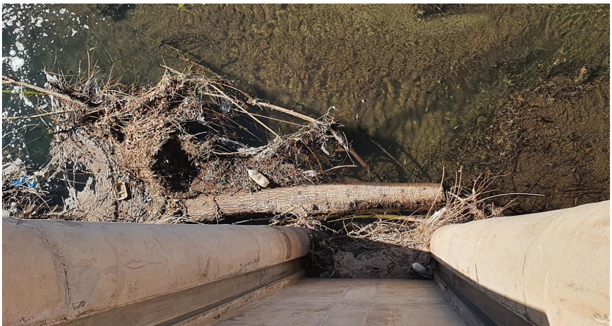
Figure 4. Top view of screen blinding (7 June 2022)
