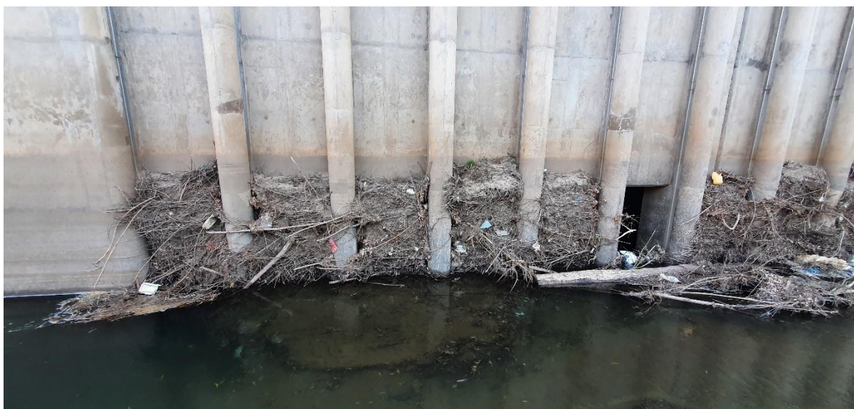
Figure 13. Densely compacted debris on the screens
